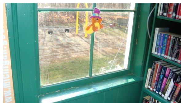
Historic Windows were painted shut, had broken panes, and were missing the original storm windows.
