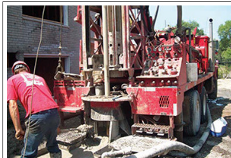
Workers drill 18 300-foot wells, which will provide geothermal heating and cooling for Rouge Woods Apartments in Detroit. With all of the green elements at the property, residents should save 30 percent to 35 percent on their electric bills.
